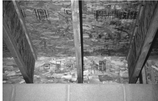
In this application, an engineered wood rim board is installed between the foundation sill plate and the floor under a wall section. The rim board matches the depth of the I-joists used in the floor framing.
